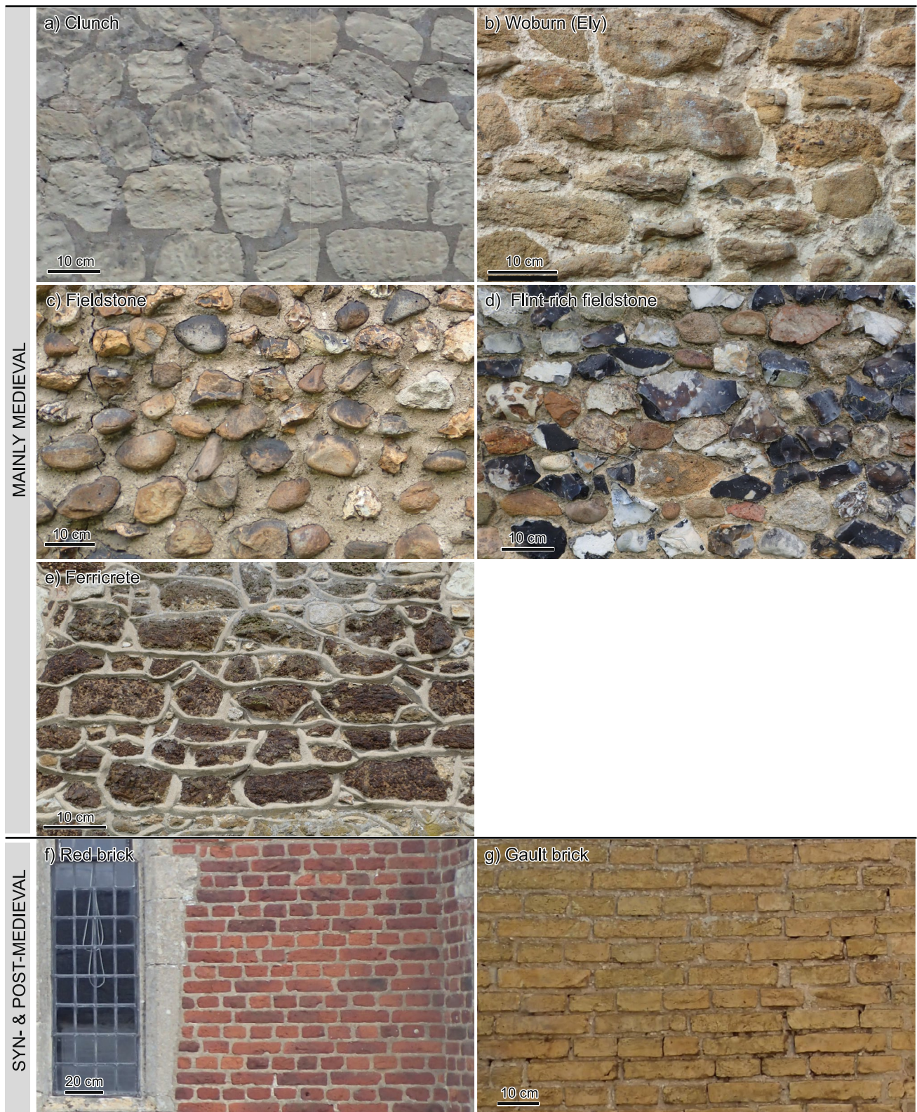
Fig. 4 Locally sourced building stones ( italicised ) used in the study area: a) Clunch block rubble, Bottisham Holy Trinity, C13 west porch; b) Ely Sandstone , Ely St Mary, early C13 north aisle; c) Fieldstone rubble, Stourbridge St Mary Magdalene, later C12 nave north;
