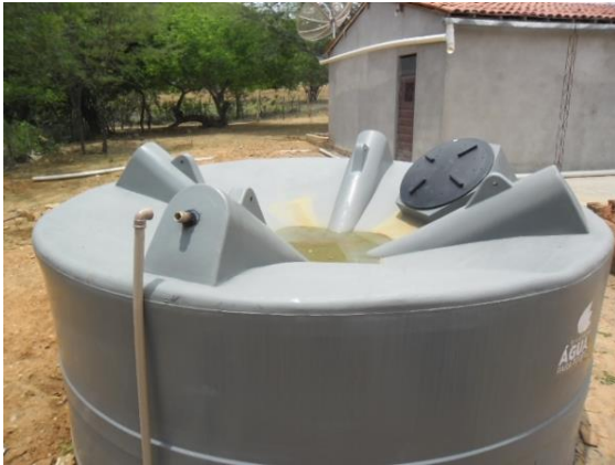
Figure 5: Collapsed polyethylene cisterna
