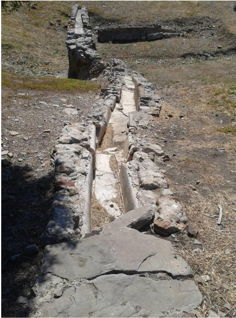
[Figure 2: aqueduct of Baelo Claudia, damaged by an earthquake and never repaired]
