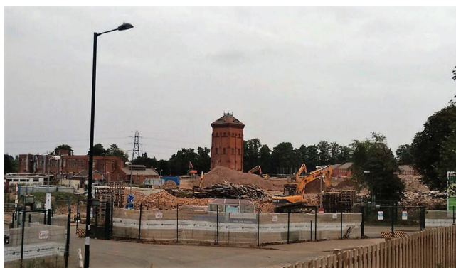
Figure 6. Selly Oak Hospital construction site. Water tower is being maintained as it is a landmark feature in the area
