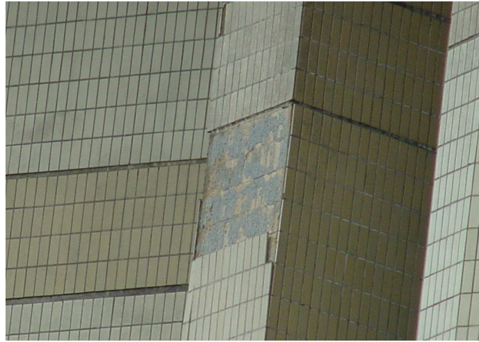
Figure 7. Debonding of plaster from substrate.
