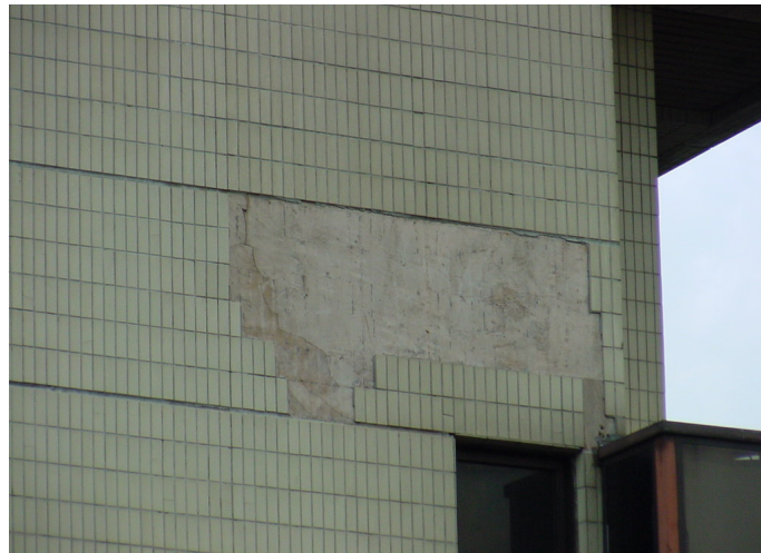
Figure 8. Debonding of tile from tile adhesive.
