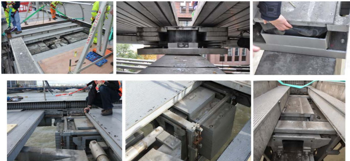
Figure 7: the inspection of the installed tuned-mass absorbers in 2012, showing (above) vertically-acting and (below) laterally-acting absorbers.
