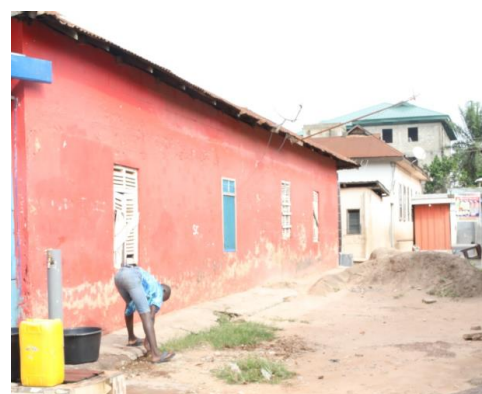
Fig. 3B. Photograph showing windows blocked to prevent theft.
